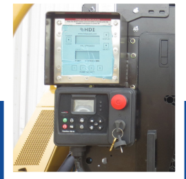
Operator's Control Station
