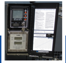
Operator's Control Station
